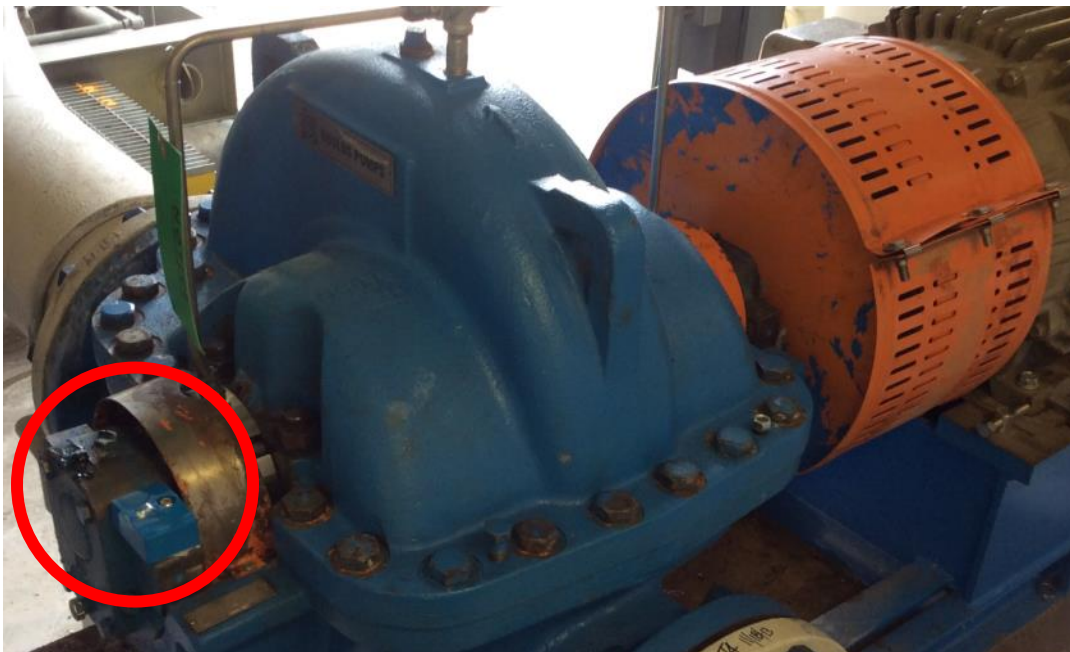
Figure 18: Double Suction , Horizontal Split case pump, mounted on thrust bearing housing
